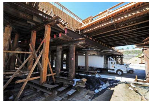
Construction continues on the I-210 bridge in Arcadia on Wednesday. The $486 million Foothill Extension from Pasadena to Azusa light rail extension has been given the go-ahead by the Metro Gold Line Foothill Extension Construction Authority. (Walt Mancini / Staff Photographer)
